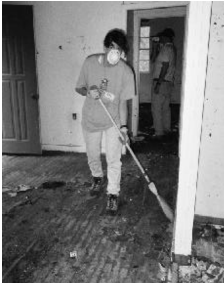
Kathy Kline "mucks out," or guts of debris, a house ravaged by the storm. Kathy described the stench as "awful!"
